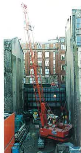
IHI CCH250 working over a shaft in the narrow streets of the City of London.
