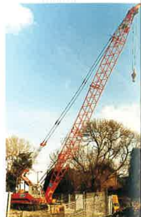
IHI CCH 350 engaged as a service crane for AMEC Piling on Thanet Way Kent.
